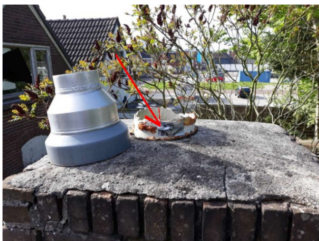
Foto 1: MM4, buis in schoorsteen
