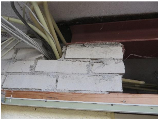
Scheurvorming in de oplegging.
